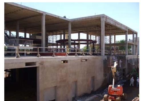
Progress: That ring in the center of the building denotes new staircase location.
